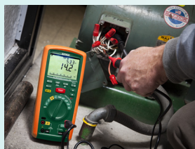
Insulation test on pump motor
